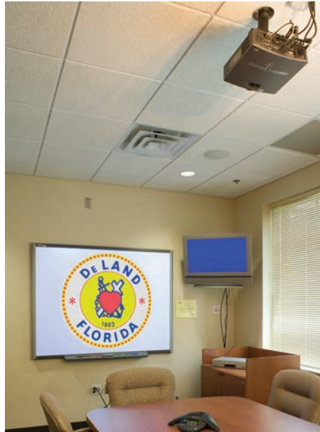
AVI-SPL also equipped three conference rooms that
